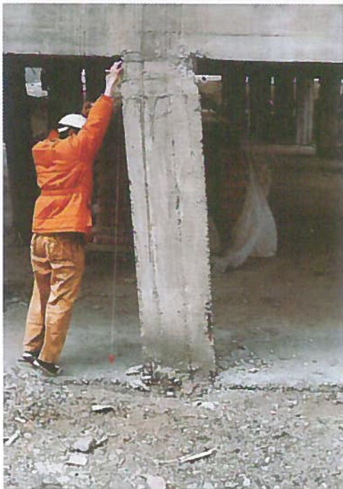
Figure D1. Sides way by Flexural Failure of Column (a)
