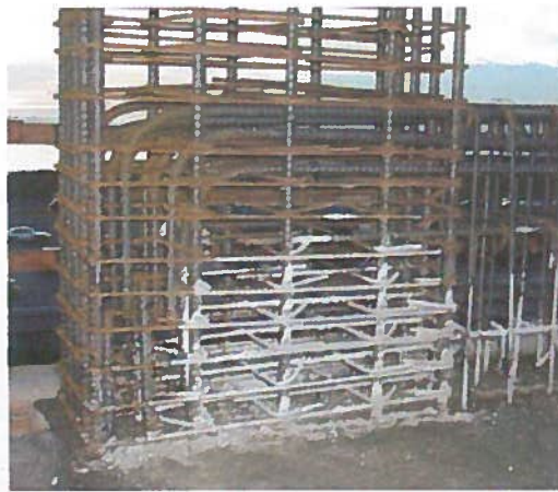
Figure 6.21 Beam-Column Joint Having Multiple Layers of Beam Reinforcement Hooked at Back Side of Joint. Note the Upturned Beam (The Slab is Cast at the Bottom Face of the Moment Frame Beam).
