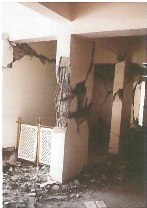
Figure D2. Shear Failure in Column (a)
