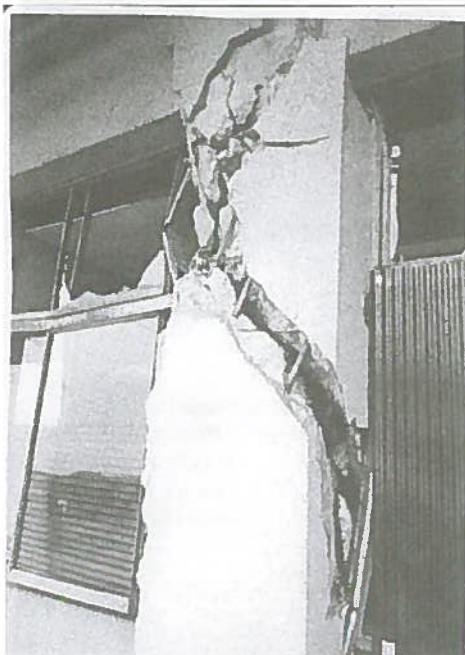
Figure D5. Shear Failure in Column (b)
