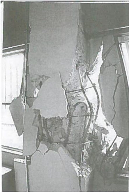
Figure D7. Shear Failure due to Short Column
