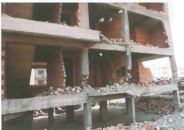
Figure D13. Exterior Brick Walls Collapse
