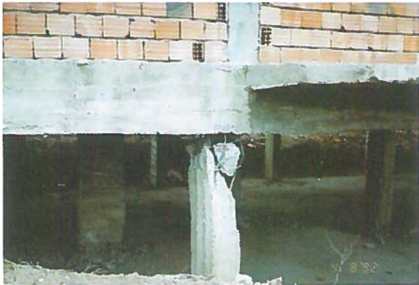
Figure D11. Ground Soft Storey Failure
