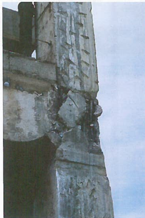
Figure D10. Shear Failure at Beam-Corner Column Joint (c)
