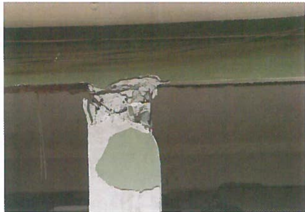
Figure D4. Shear & Flexural Failure at Column Top
