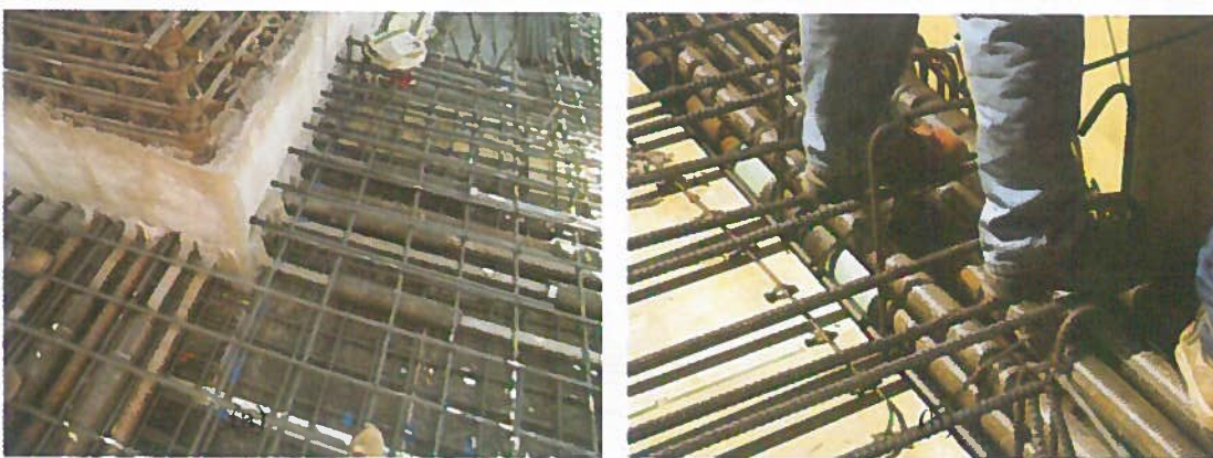
Figure 6.47 Collector Detailing, (A) Collector Connection to Shear Wall Boundary Zone; (B) Beam for Large Collector
