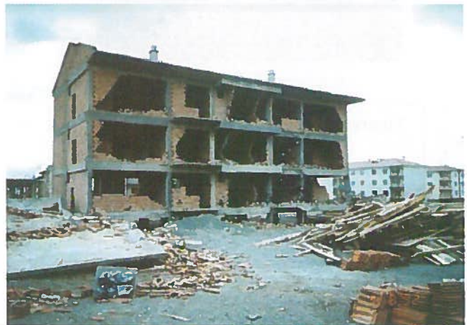
Figure D14. Exterior Brick Walls Collapse
