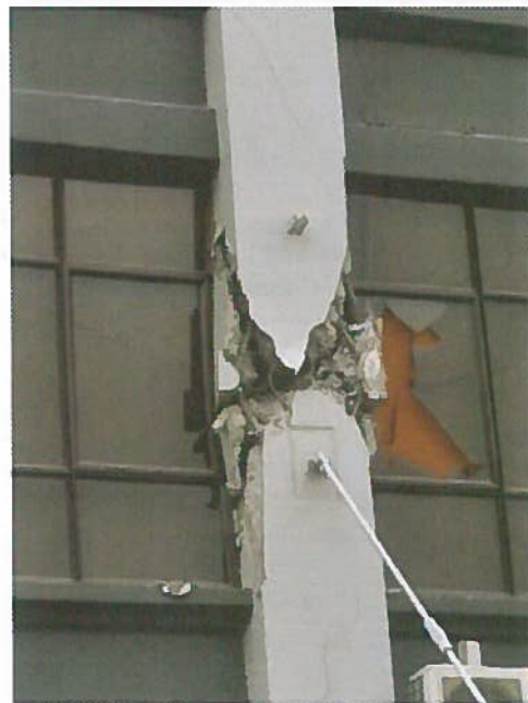
Figure D6. Shear Failure of Column due to Short Column
