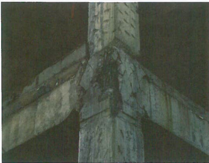
Figure D9. Shear Failure at Beam-Corner Column Joint (b)
