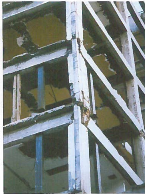
Figure D8. Shear Failure at Beam-Corner Column Joint (a)
