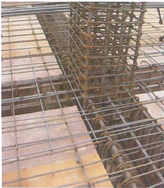
Figure 6.19 Beam-Column Joint with Beam Corner Bars Swept to Inside of Column Corner Bars.
