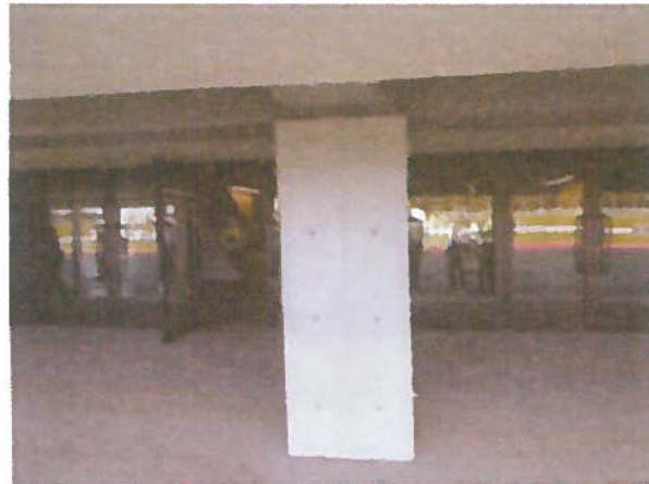
Column Jacketing with Steel Plate in Stadium at Chiba City (After Construction)
