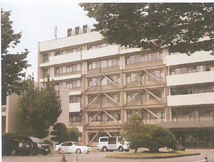
External Steel Frame Bracing is applied as retrofitting in a building of Tohoku University
