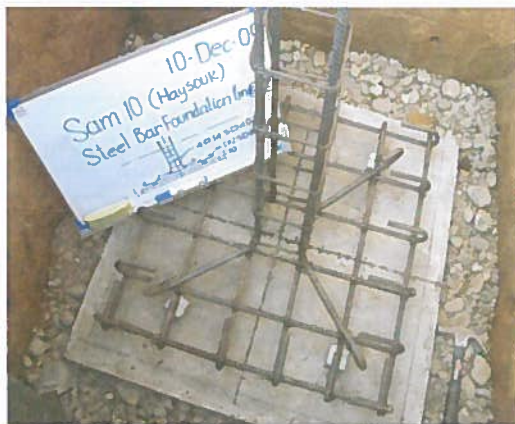
PHOTO 3: Check number of bar, size, pitches, tied each bar Setting correctly in the center a line
