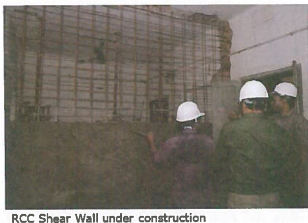
Figure 4.2.7 Photograph of RC Shear Wall Insertion during Construction of Pilot Work of CNCRP
