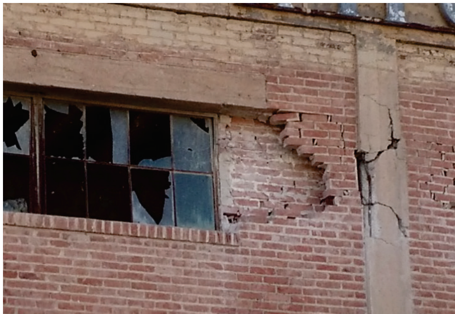
Figure O-8 Damage in infill panel with opening causing shear failure in bounding column (Yousefianmoghadam and Stavridis, 2018).
