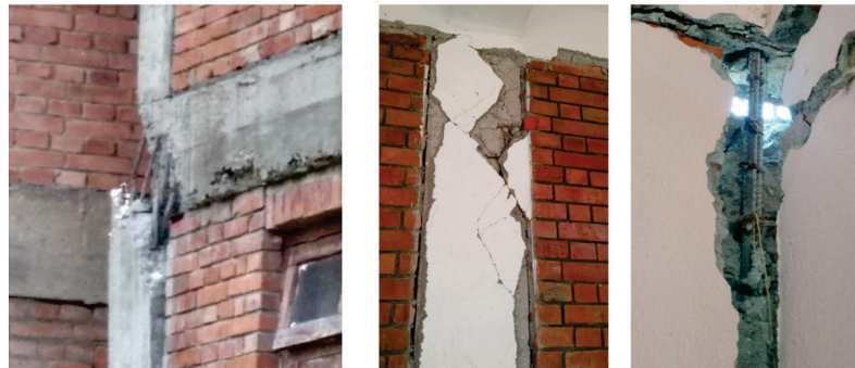
Figure O-23 Damage to an infilled frame building, showing severely damaged columns, but no collapse. Infill panels are likely carrying significant portion of the gravity loads (Bose et al., 2017).
