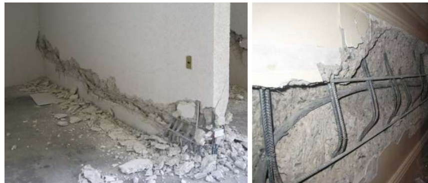
Concrete crushing and buckling of longitudinal reinforcement initiating at wall boundaries and propagating along the length of wall segments
